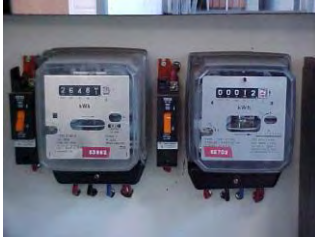
Conventional Electricity meter
